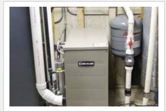
New GV906 Boiler
